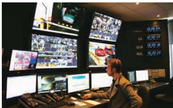
Central monitoring system, Care Assist
